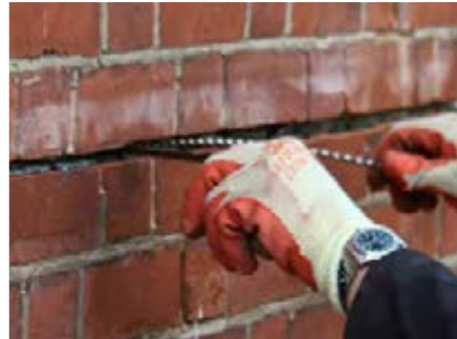
STEP 4 Using a finger trowel, or similar, push the HeliBar into the grout to obtain good coverage.
