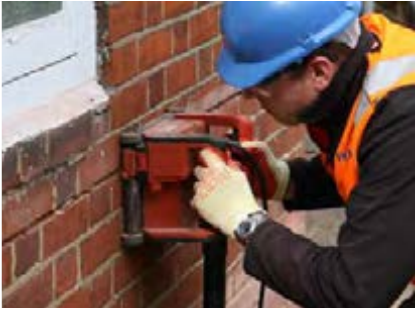
STEP 1 Cut slots into the masonry to a minimum of 500mm either side of the crack and to the specified depth.
