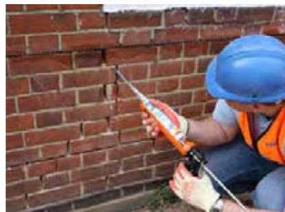
STEP 6 Repoint the mortar bed with a suitable mortar and make good the vertical crack with an epoxy-based weatherproof filler, e.g. CrackBond TE.
