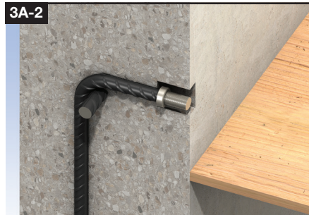
Remove the formwork and polystyrene and screw the locknut onto the fixed bar.
