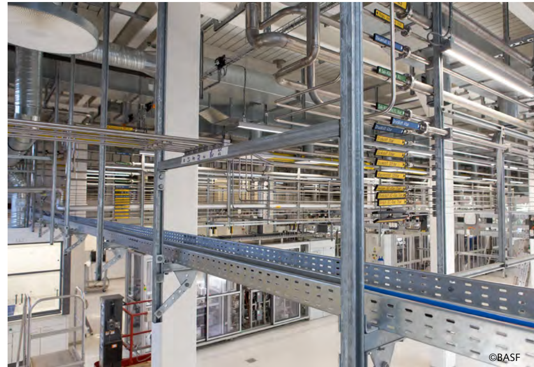
HALFEN Powerclick used as a standardized support system for all utility systems in BASF's new Research Centre M400.
