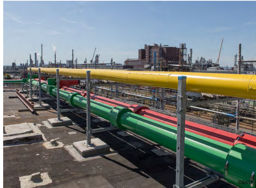
Support for the steam and condensate pipes using HALFEN Powerclick.
