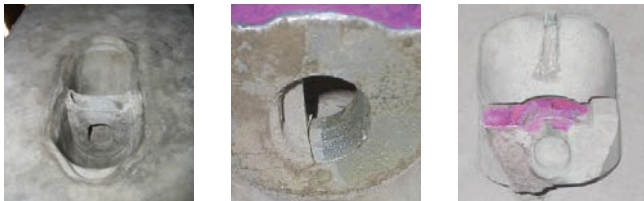
Examples of blocked lifting holes
